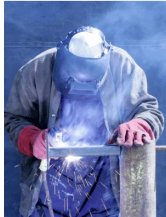
No extraction system used
