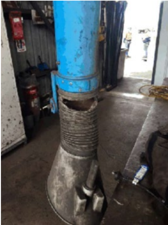
Damaged fume extraction unit
