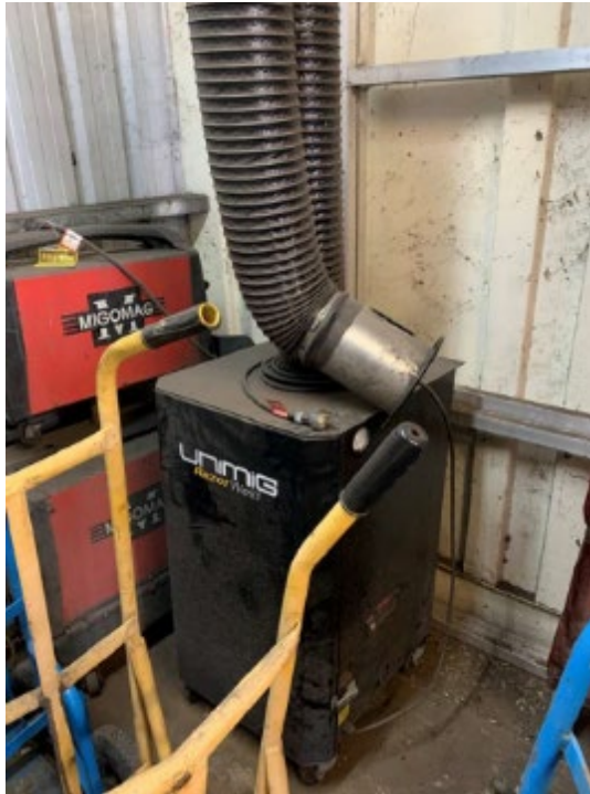
Disused fume extraction unit
